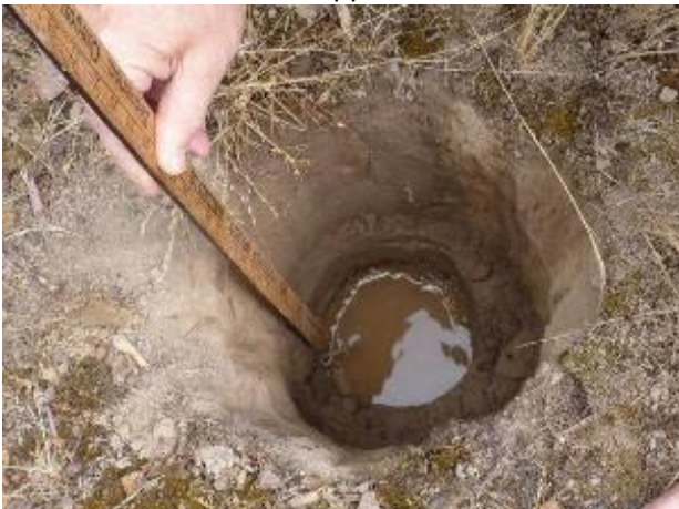
Figure B-2. A shovel was used to dig most of the way then a 6" diameter post hole digger was used to reach the proposed bottom elevation of a rain garden. Measure the drop in water from a known, stable marker.
