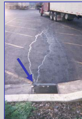
Oil from parking lot entering storm system
